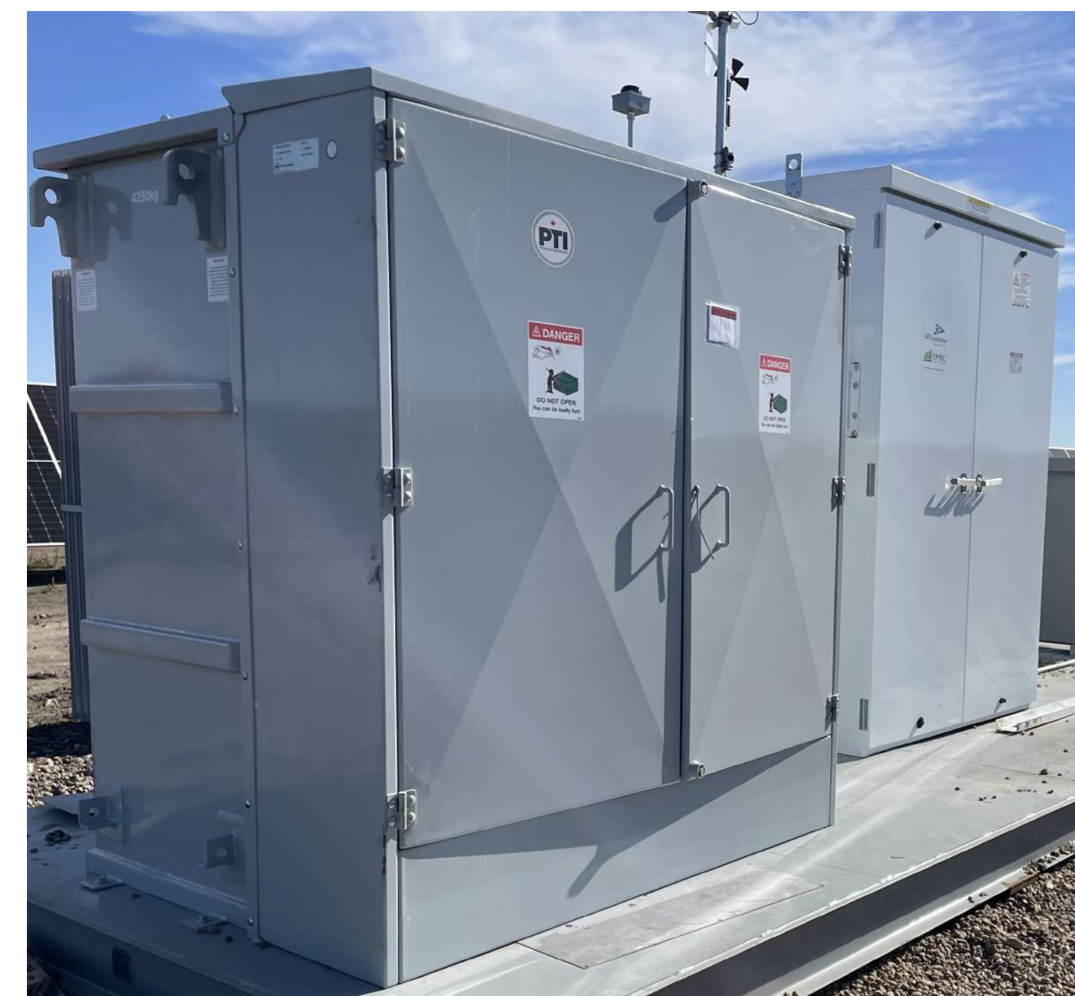
Figure 2 - 44kV HV Step Up Transformer (Approximate Dimensions - Height: 8.5ft, Width: 12 ft, Depth: 8.5ft)
